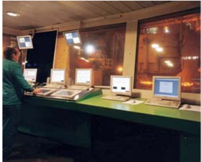
▲ Electric furnace control panels continuously monitor the steel processing.
